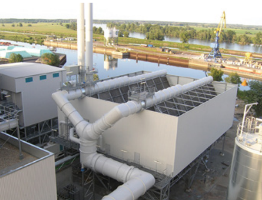
Figure 1: A-frame at existing plant
