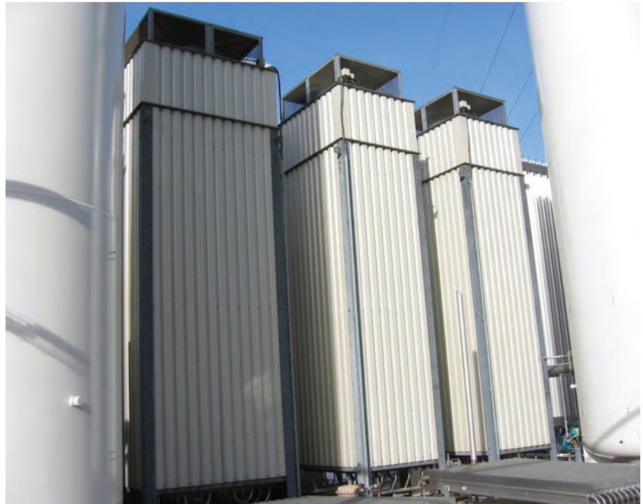
Fig. 2: Gas evaporation towers with Whizz-Wheel® fans; 50 percent of the number of towers
