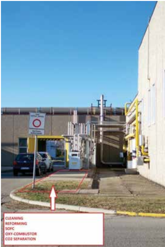
Plant site of the Demonstration in SMAT (Torino, Italy)
