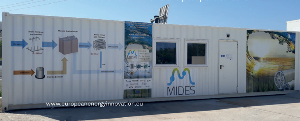
Outside view of the ceramic membrane pilot plant container
