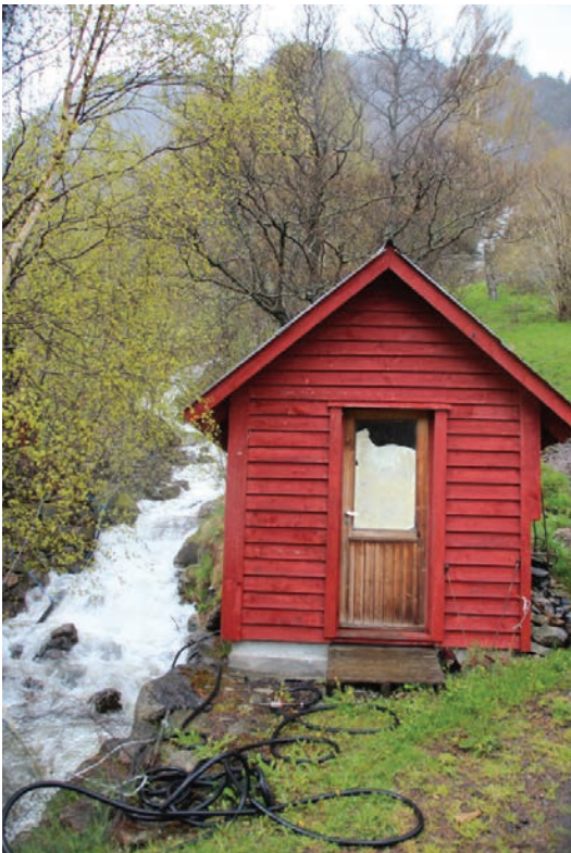
Mr. Leidulf Bogstad on the outside of one of his powerplants, beautifully located by the fjord. (Below) The size makes no difference. Even in a small hut you can find room for a generator.
