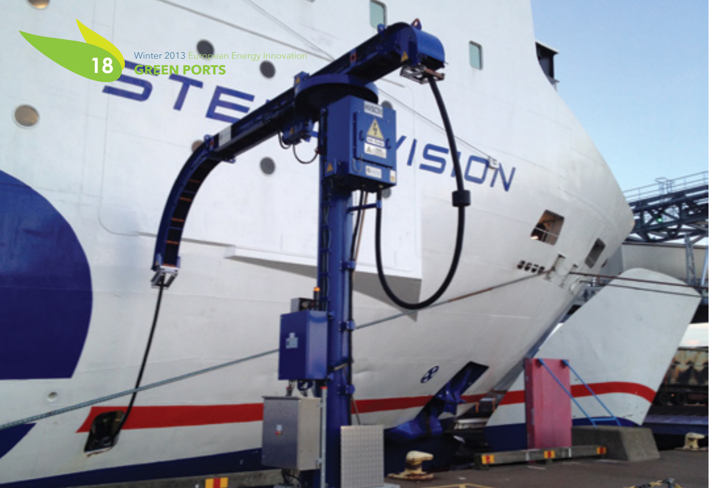
Stena Line ferry connected to on-shore power supply in the Port of Karlskrona, Sweden
